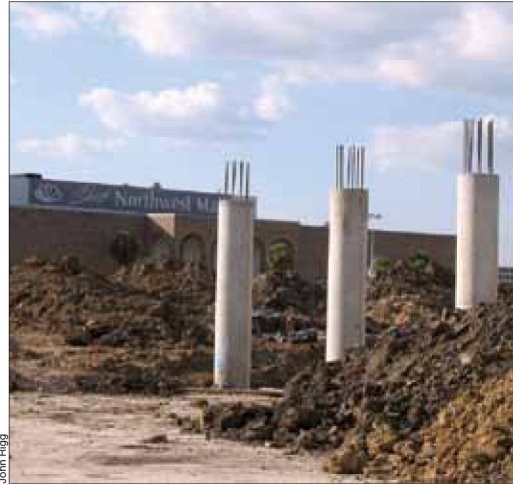
The Hwy. 290 expansion project has displaced parking spaces at the Northwest Mall near Loop 610.
